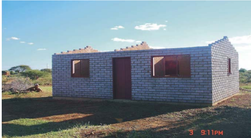
Fig. 4. Incomplete house: Tswaing Local Municipality
